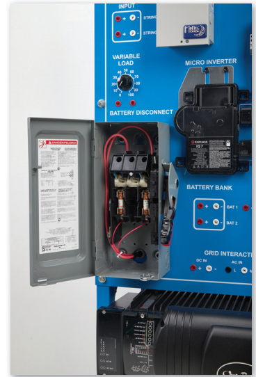
Micro-Inverter & Battery Disconnect on 950-SPT1
